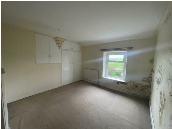
With built in storage and two radiators.
